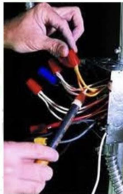
Always test a circuit to make sure it is de-energized before working on it.
